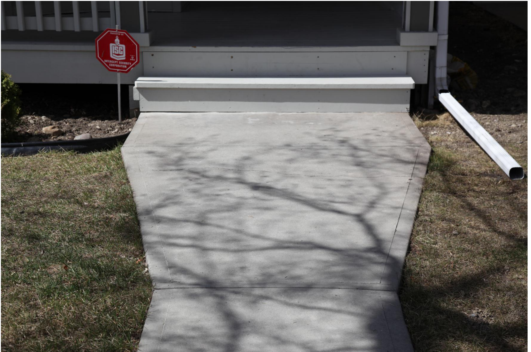
Formerly sunken sidewalks lifted, shimmed and no longer a tripping hazard. (North Unit)
