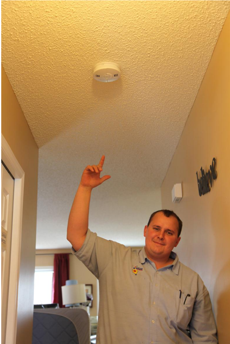
Derek from 4-Star Electric ensures us that replacement of all Smoke Alarms means both South and North Suites are safe!
