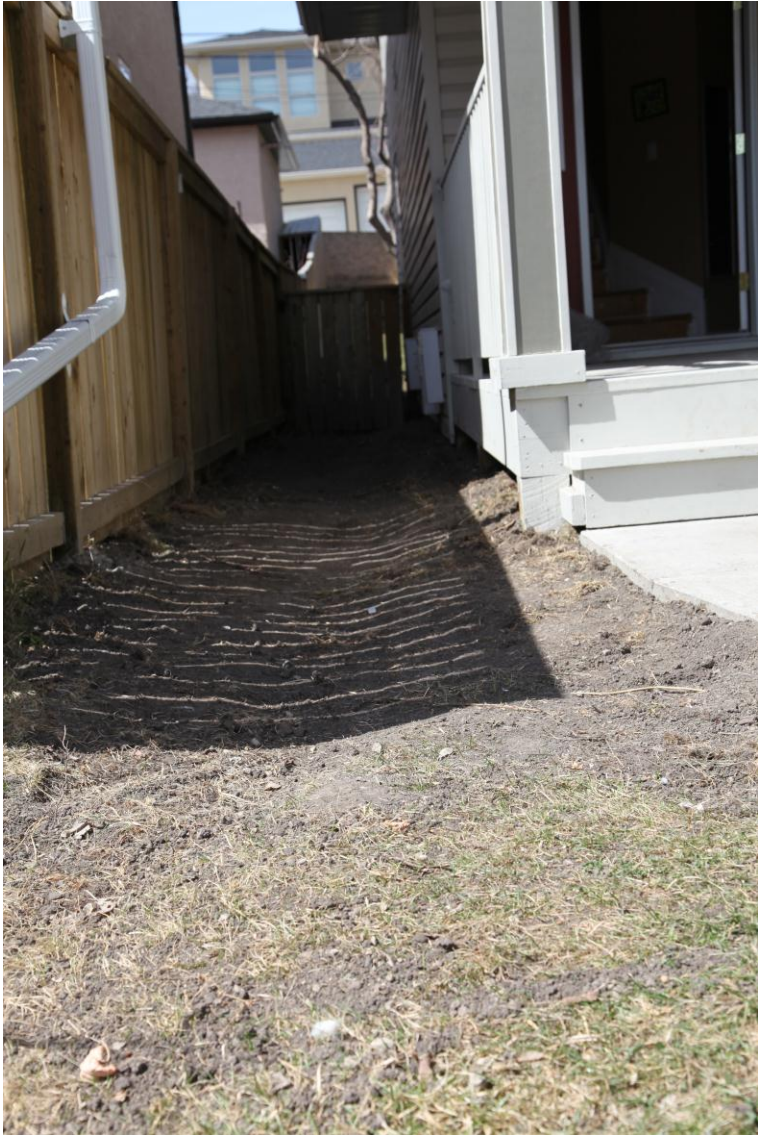
South side yard now has drainage swale and grass planted to ensure moisture drains away; not towards foundation.
