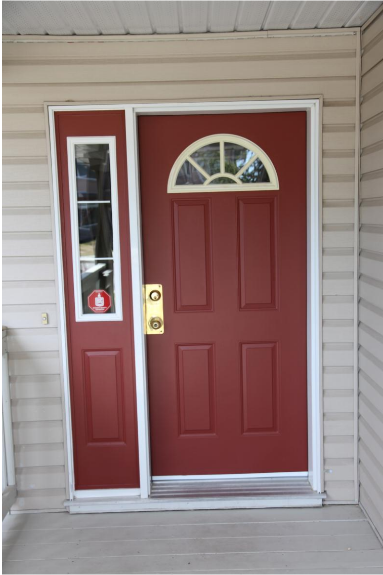
Split Jamb repair completed, new Threshold installed and Crisply painted; makes this door look like brand new!
