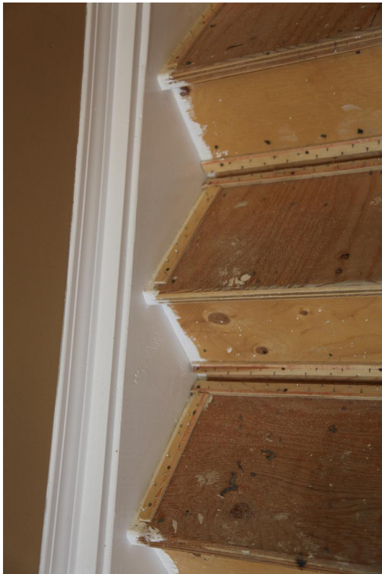
Stair Stringers get a repairs and a fresh coat of paint before carpet is installed.
