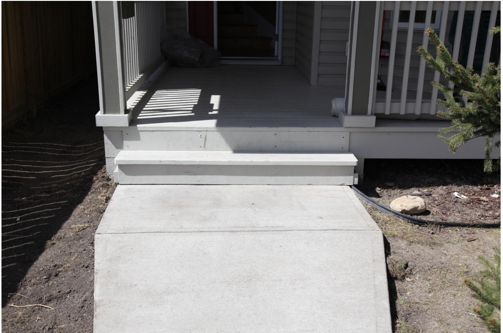
Formerly sunken sidewalks lifted, shimmed and no longer a tripping hazard. (South Unit)
